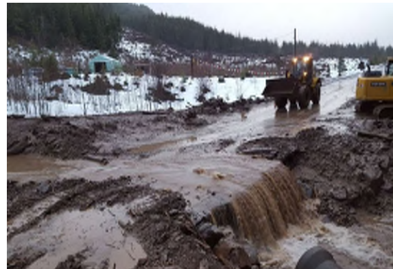
Highway 7 after a massive mudslide in February of 2017
