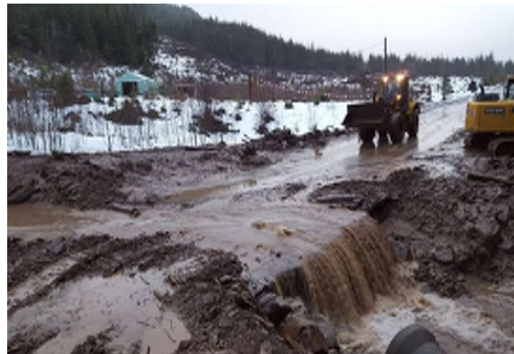
Highway 7 after a massive mudslide in February of 2017
