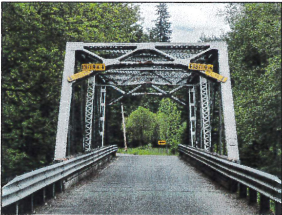
Ferrier Bridge #93 is posted with height restrictions
