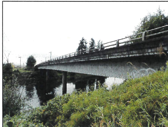
Galvin Bridge #75, built in 1969 is a bridge that requires an underwater inspection every five years
