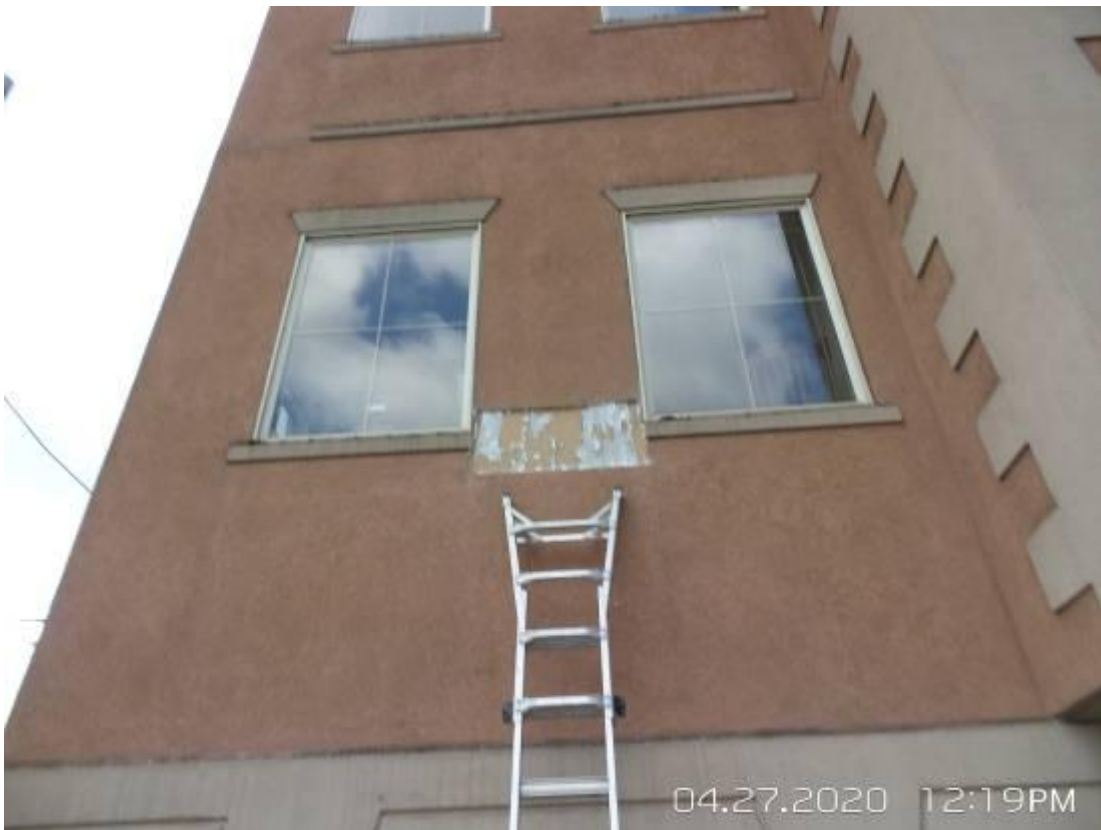
8. No WRB installed at any opening; north elevation shown.
