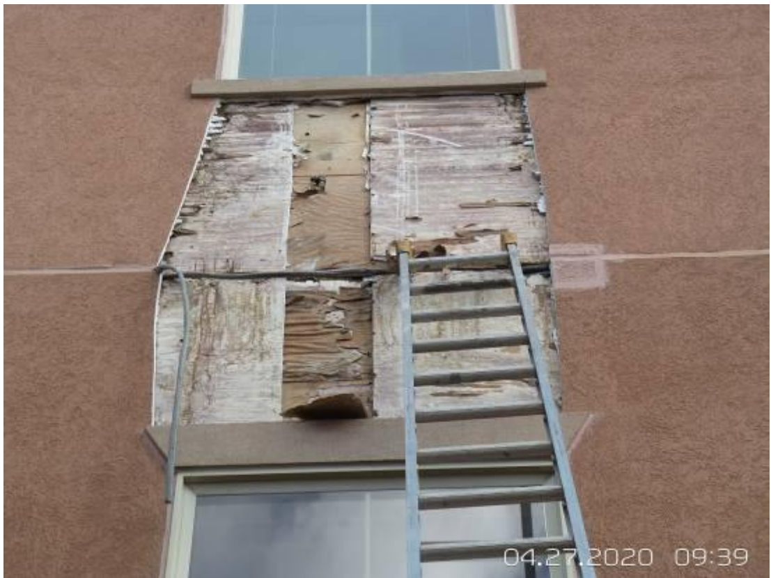
30. Opening 3 – the paper facer at the second layer of gypsum sheathing was delaminated
