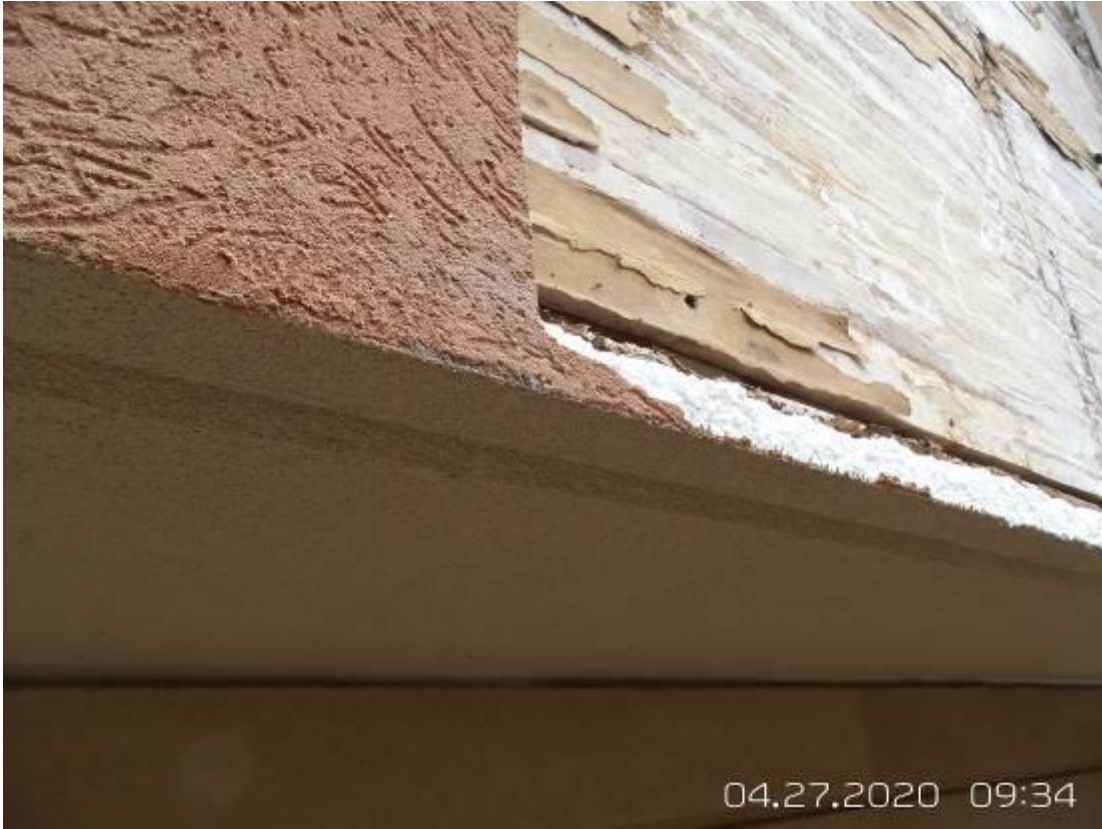
19. Opening 2 – no weeps or gap for drainage of incidental moisture was provided as part of the cladding assembly.
