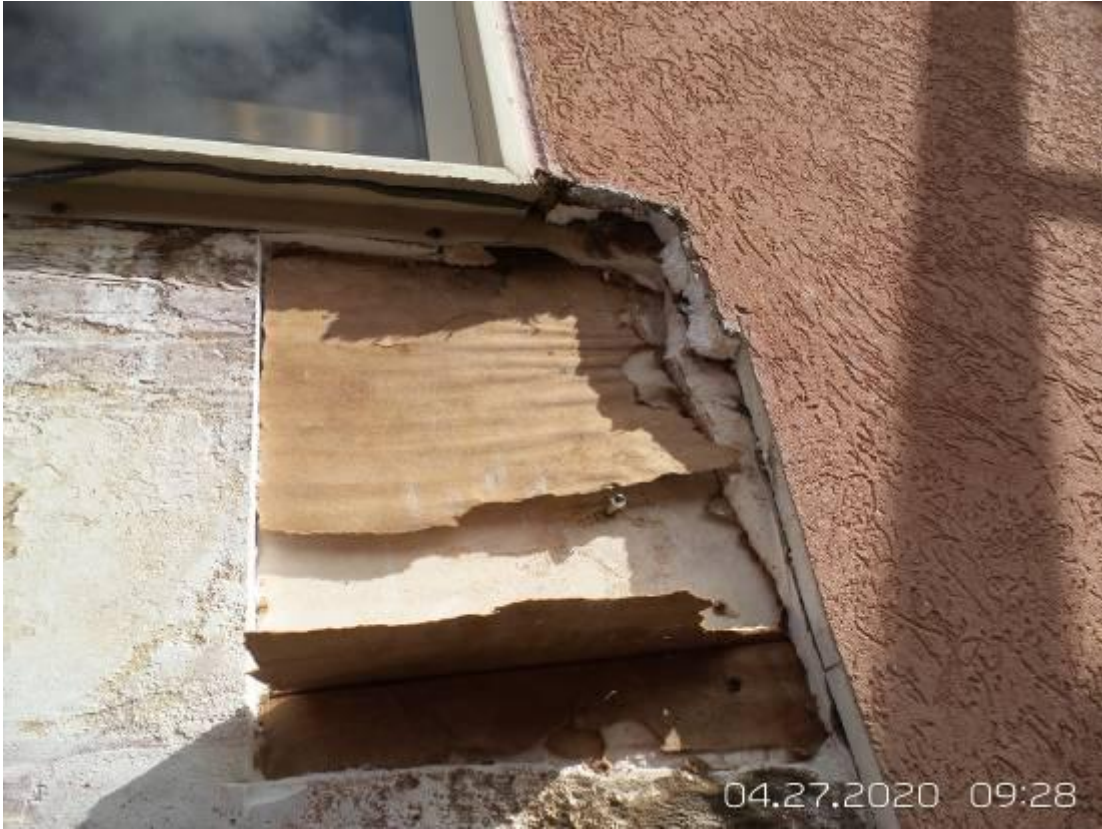
23. Opening 2 – the paper facer at the second layer of gypsum sheathing was delaminated.
