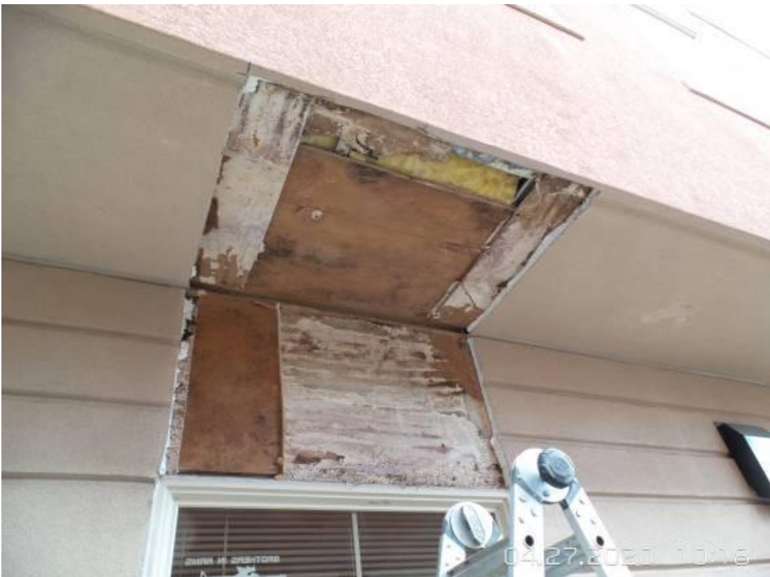
36. Opening 4 – staining of second layer of gypsum sheathing was observed.
