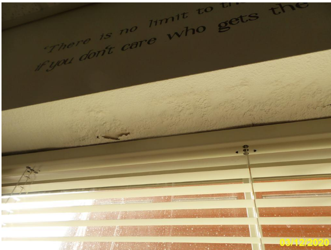
40. Opening 4 – staining and peeling paint at the interior finish above window head.
