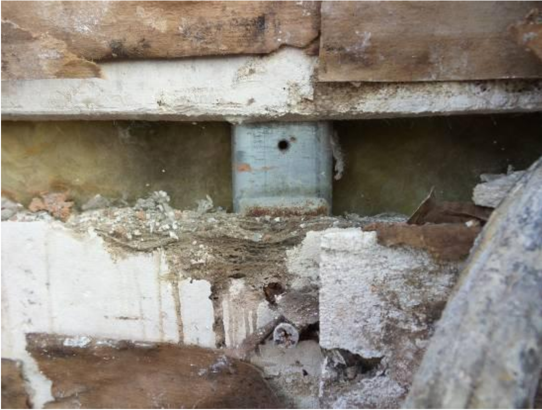
31. Opening 3 – surface corrosion of steel stud framing was observed.
