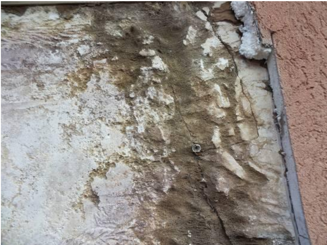
22. Opening 2 –the gypsum sheathing core was cracked and deteriorated.
