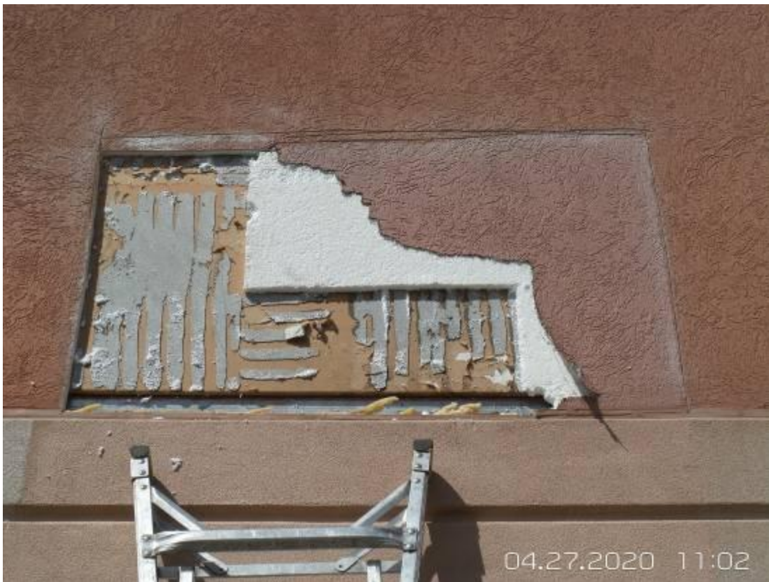
42. Opening 5 – insulation board was adhered to gypsum sheathing, no deterioration of the gypsum sheathing was noted at the opening.
