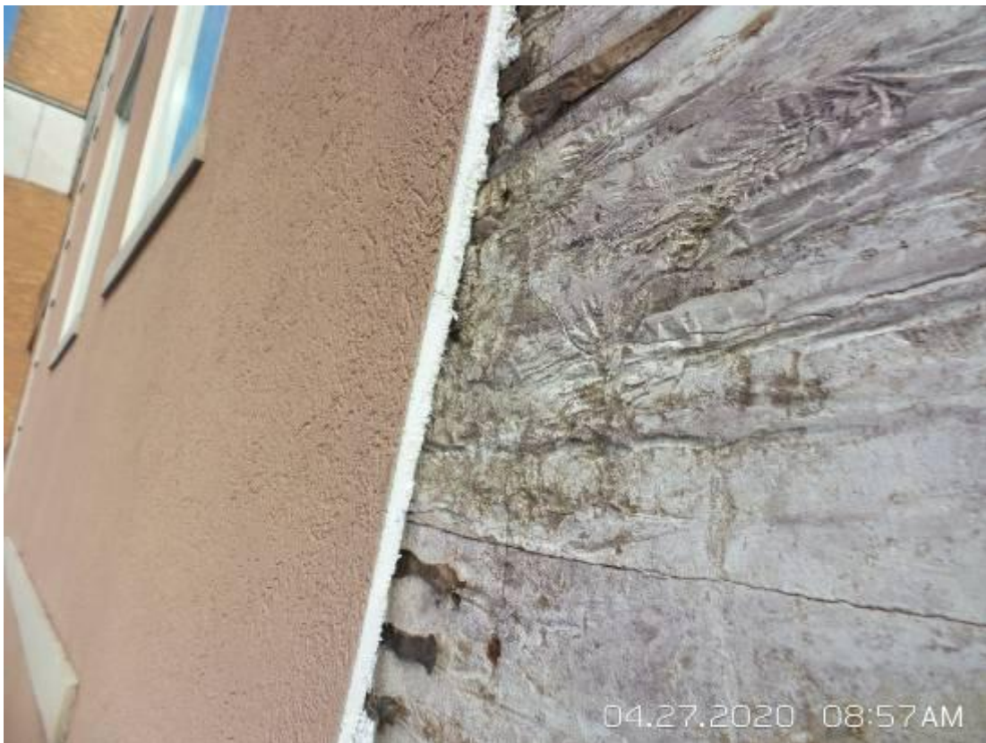
28. Opening 3 –the gypsum sheathing core was deteriorated.
