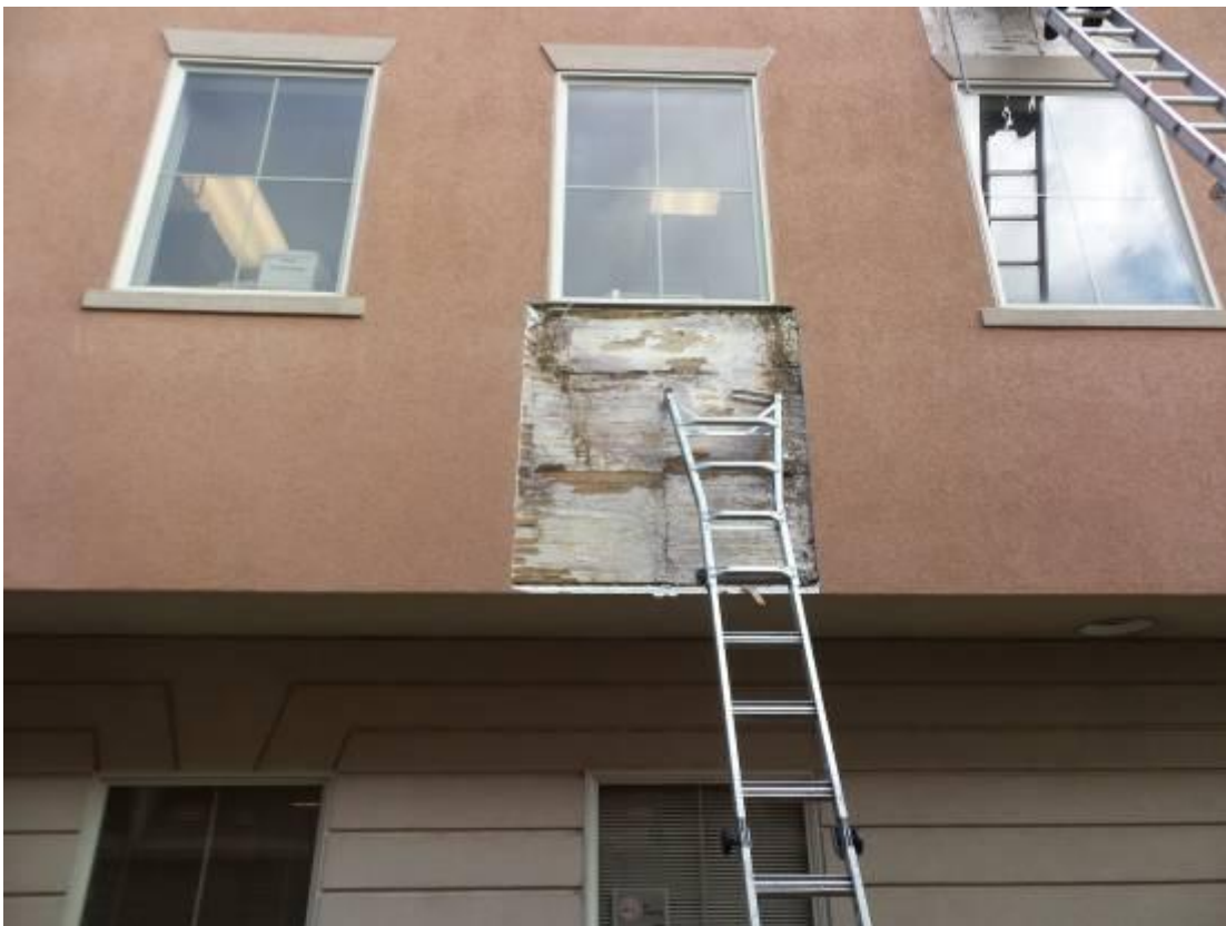
18. Opening 2 – gypsum sheathing was deteriorated across the opening area.
