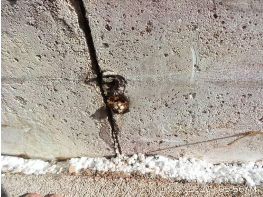
29. Opening 3 – corroded fasteners were observed across the opening.
