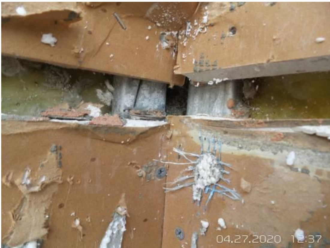
56. Opening 8 – no corrosion of steel stud framing was observed.
