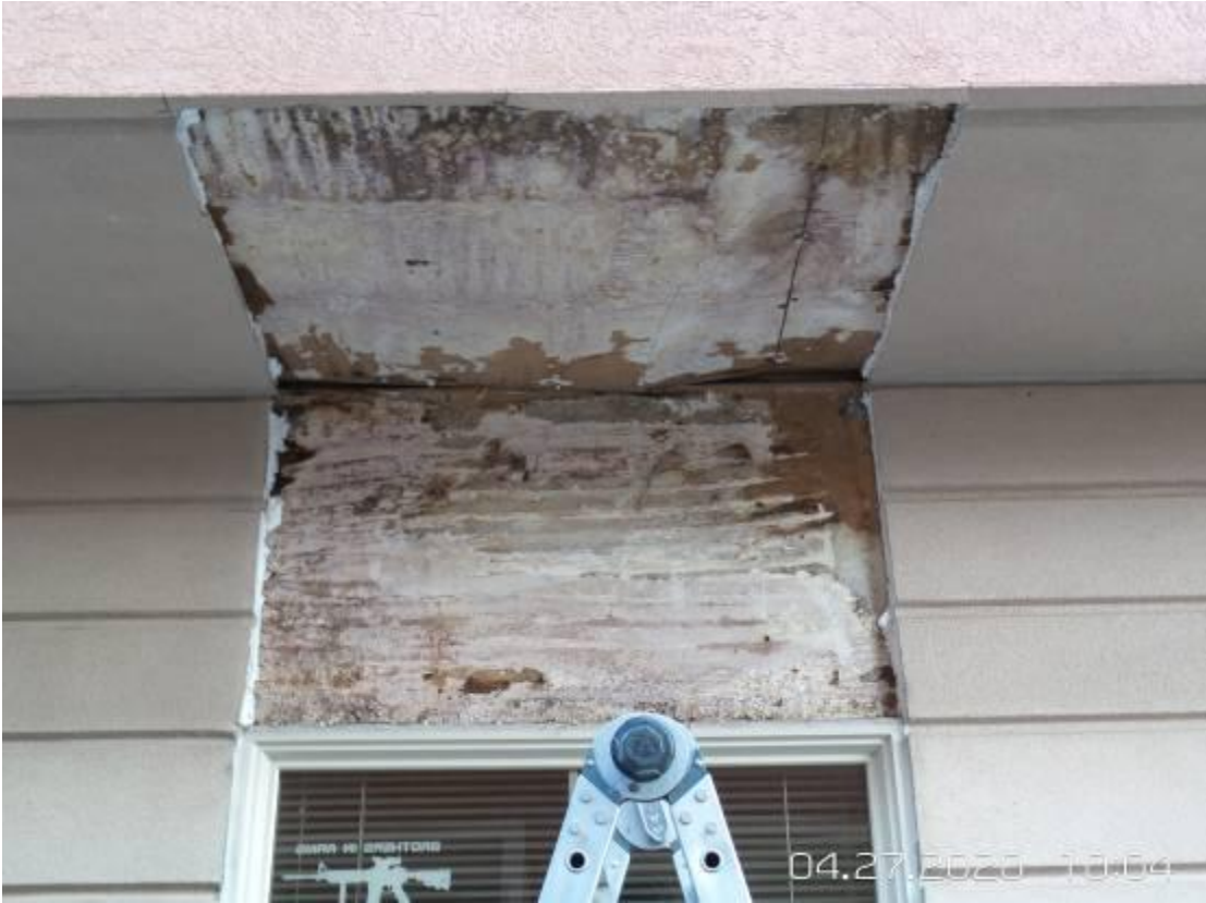
35. Opening 4 – gypsum sheathing was deteriorated and delaminated across opening.
