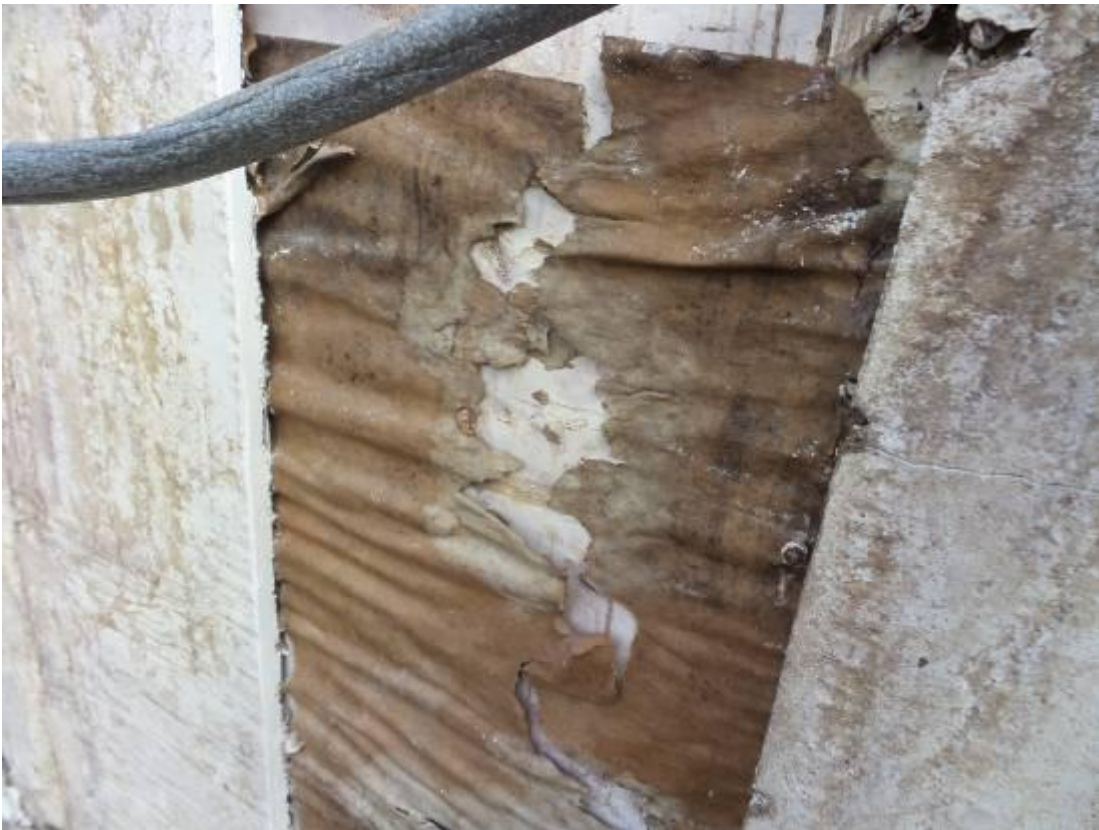
32. Opening 3 –the paper facer of the gypsum sheathing was delaminated and deteriorated.
