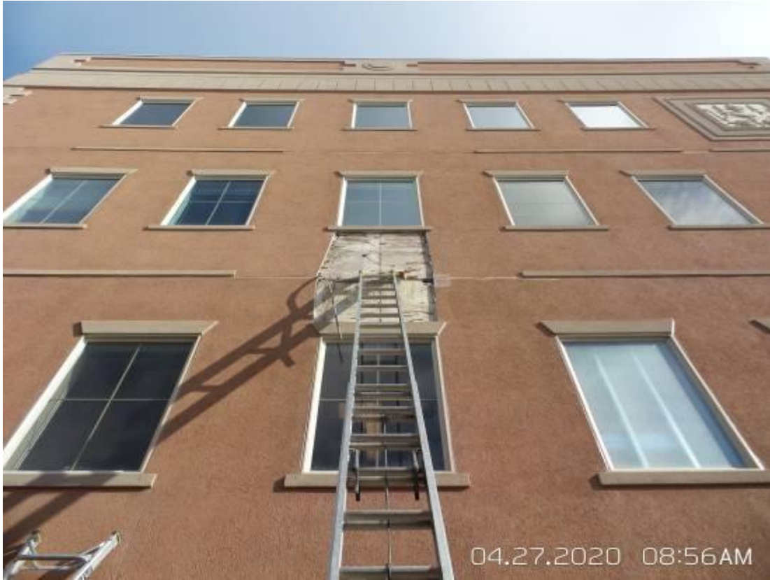
27. Opening 3 – gypsum sheathing was deteriorated across the opening area.
