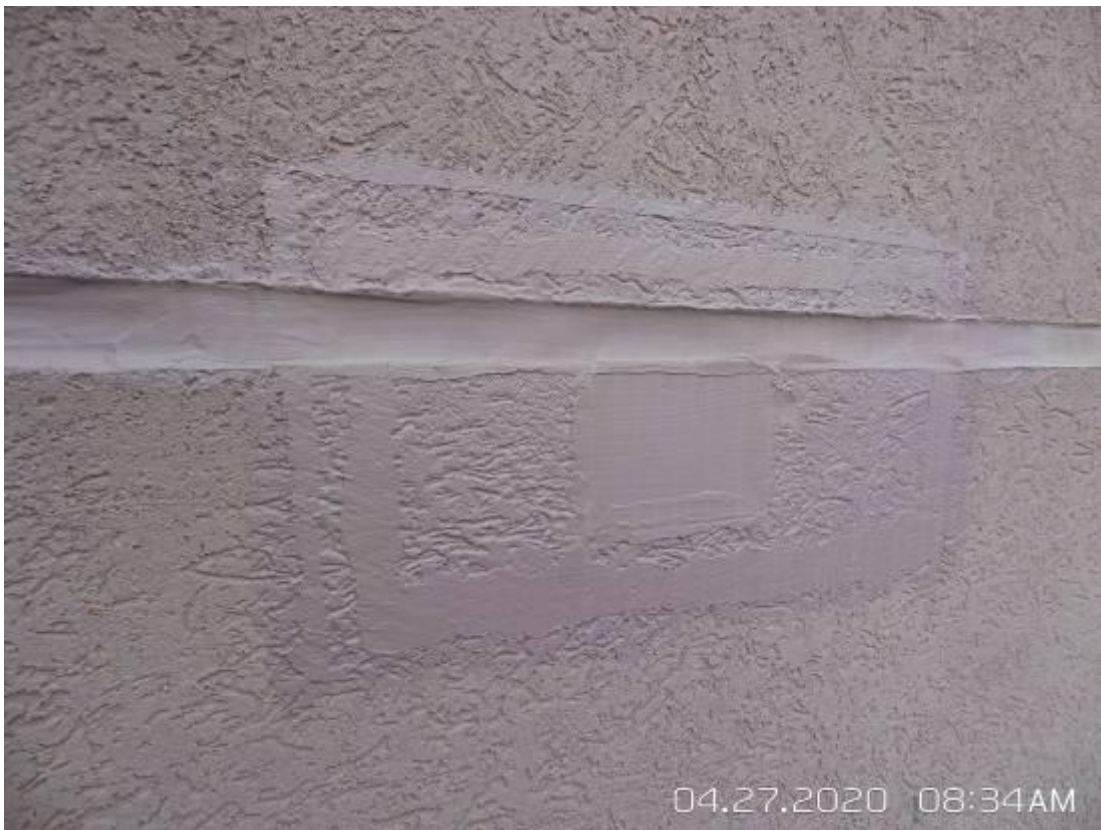
26. Opening 3 – previous repair observed at control joint between second and third floors.
