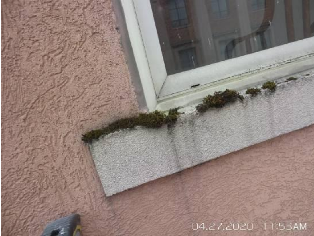
51. Opening 7 – organic growth observed on all horizontal trim accents.
