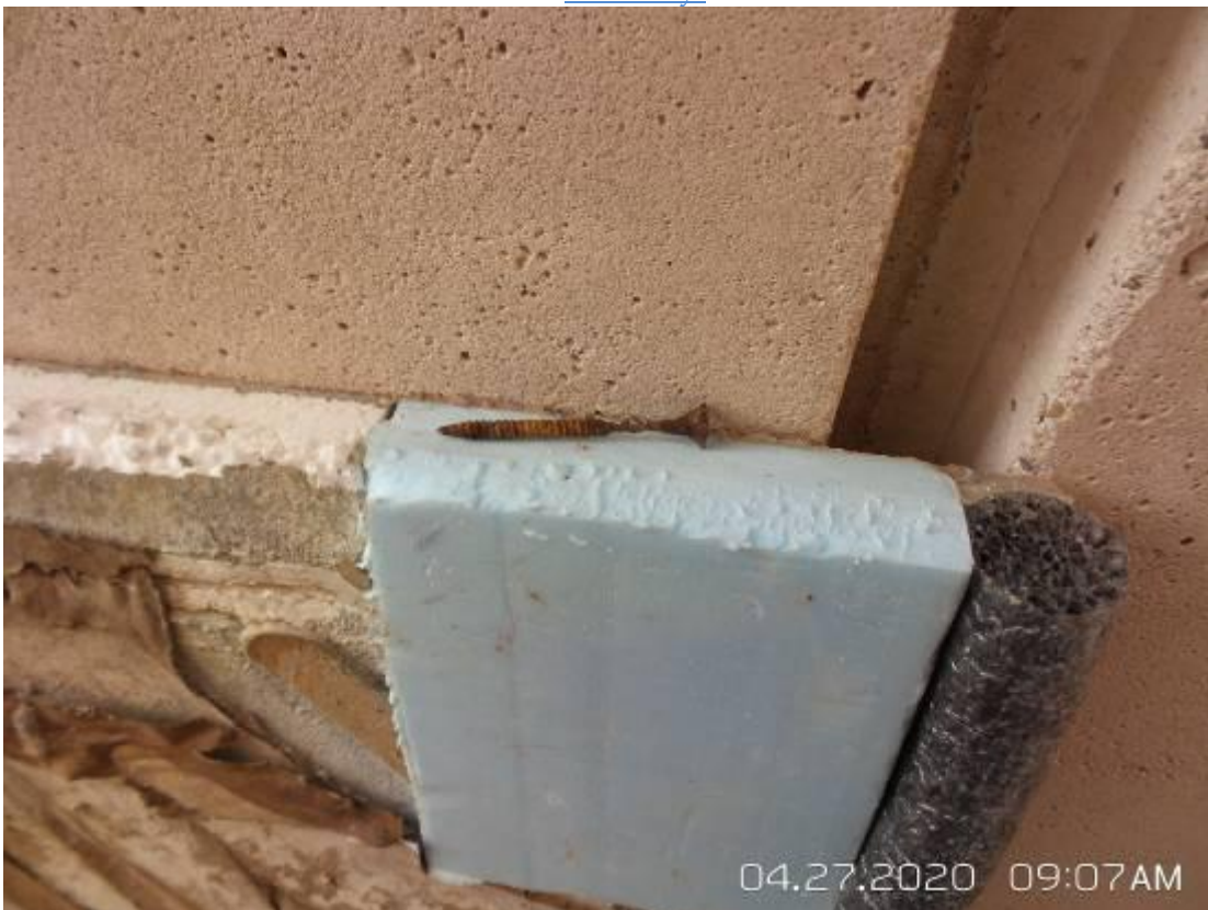
20. Opening 2 – insulation board fastener deterioration was noted.
