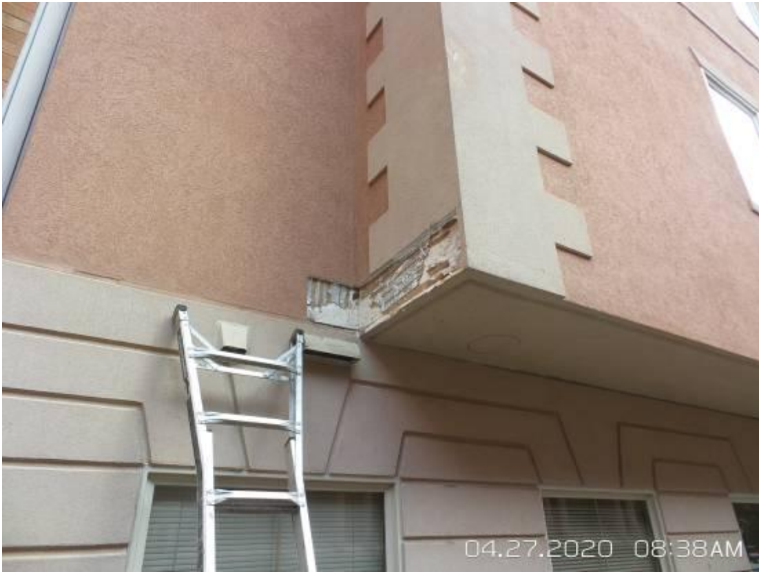
13. Opening 1 –the paper facer of the gypsum sheathing was delaminated primarily at the base of the opening.
