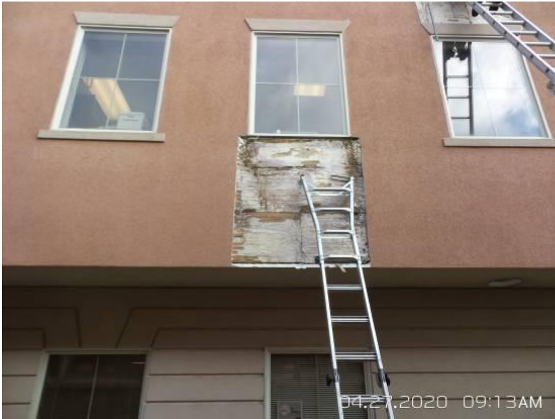
7. No WRB installed at any opening; south elevation shown.
