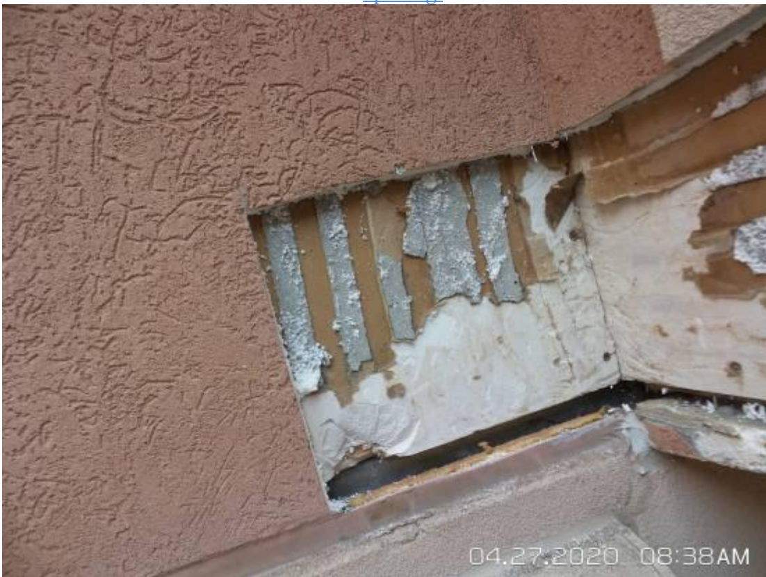
14. Opening 1 – gypsum sheathing paper facer was adhered at the top of opening, but was delaminated at the bottom of opening.
