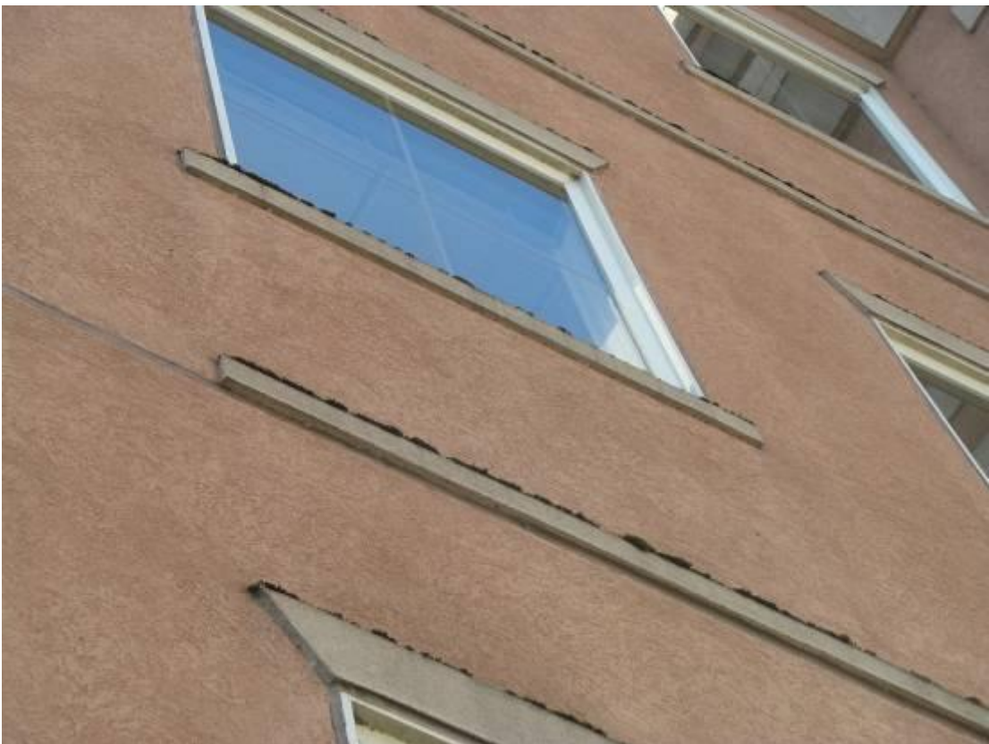
6. Organic growth observed on north elevation on horizontal trim surfaces.
