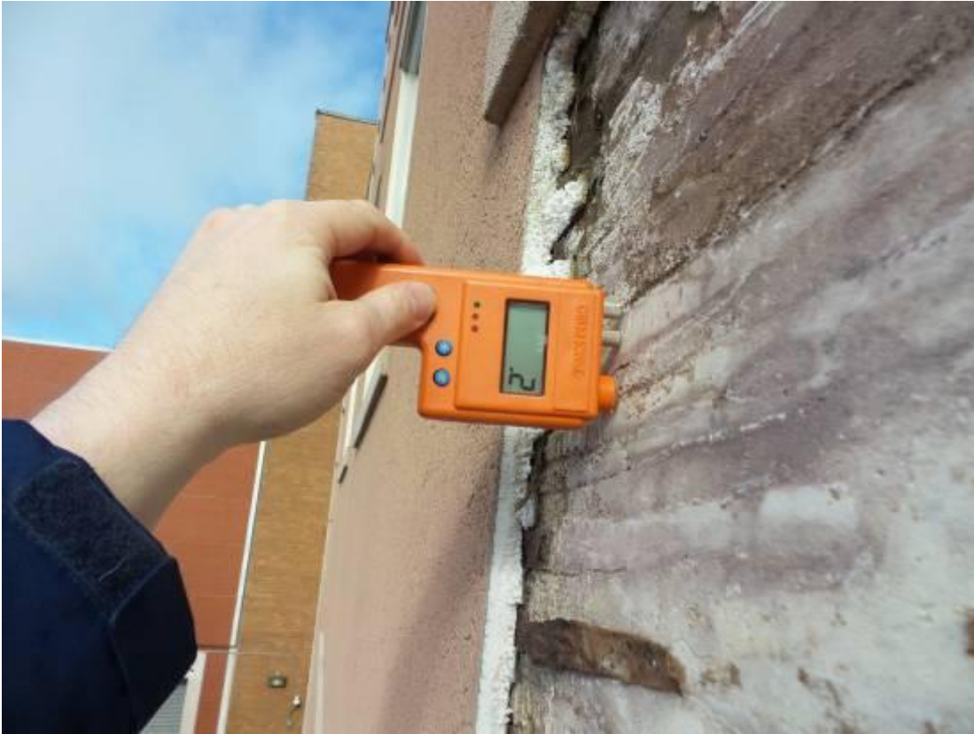
33. Opening 3 – moisture content readings of the gypsum sheathing were normal (0.1% - 0.2%).
