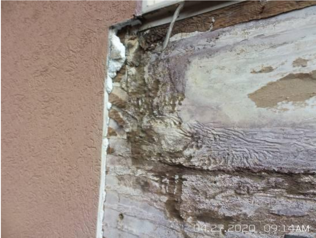
21. Opening 2 – the gypsum sheathing core was deteriorated below the window sill.
