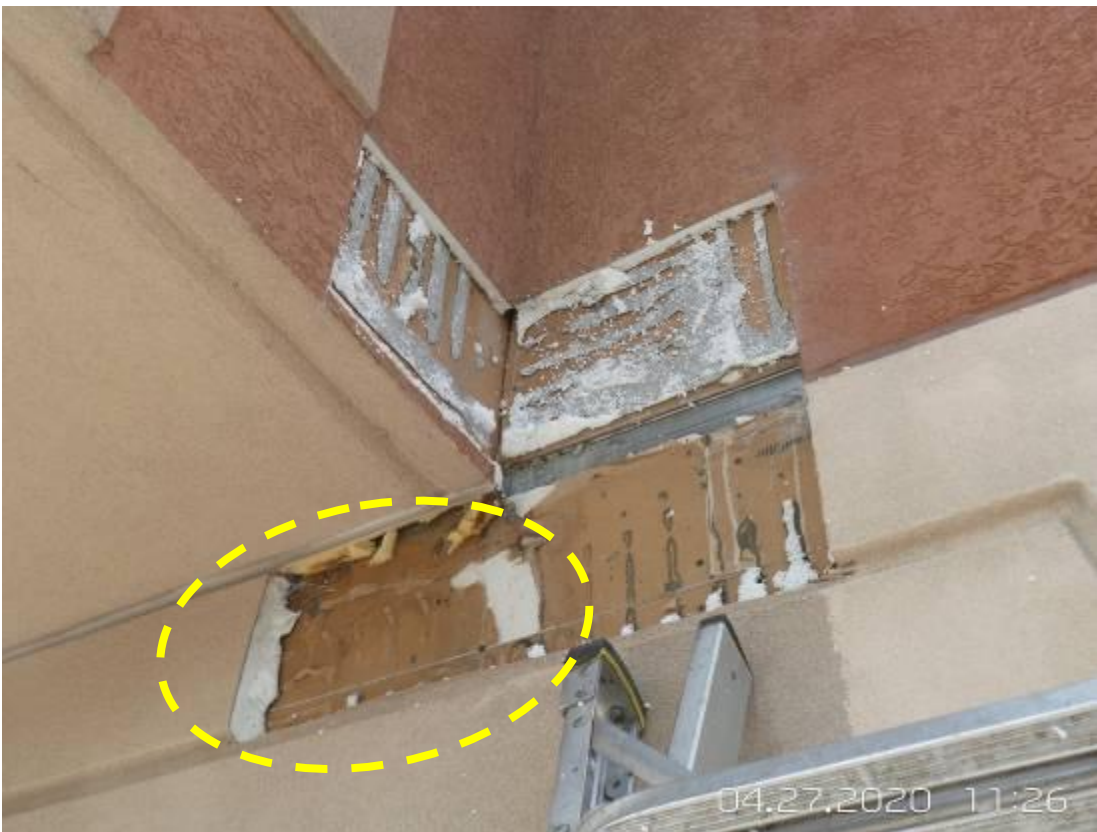
46. Opening 6 – insulation board was adhered to the gypsum sheathing above the soffit; however, the insulation board was not adhered below the soffit (see circled area).
