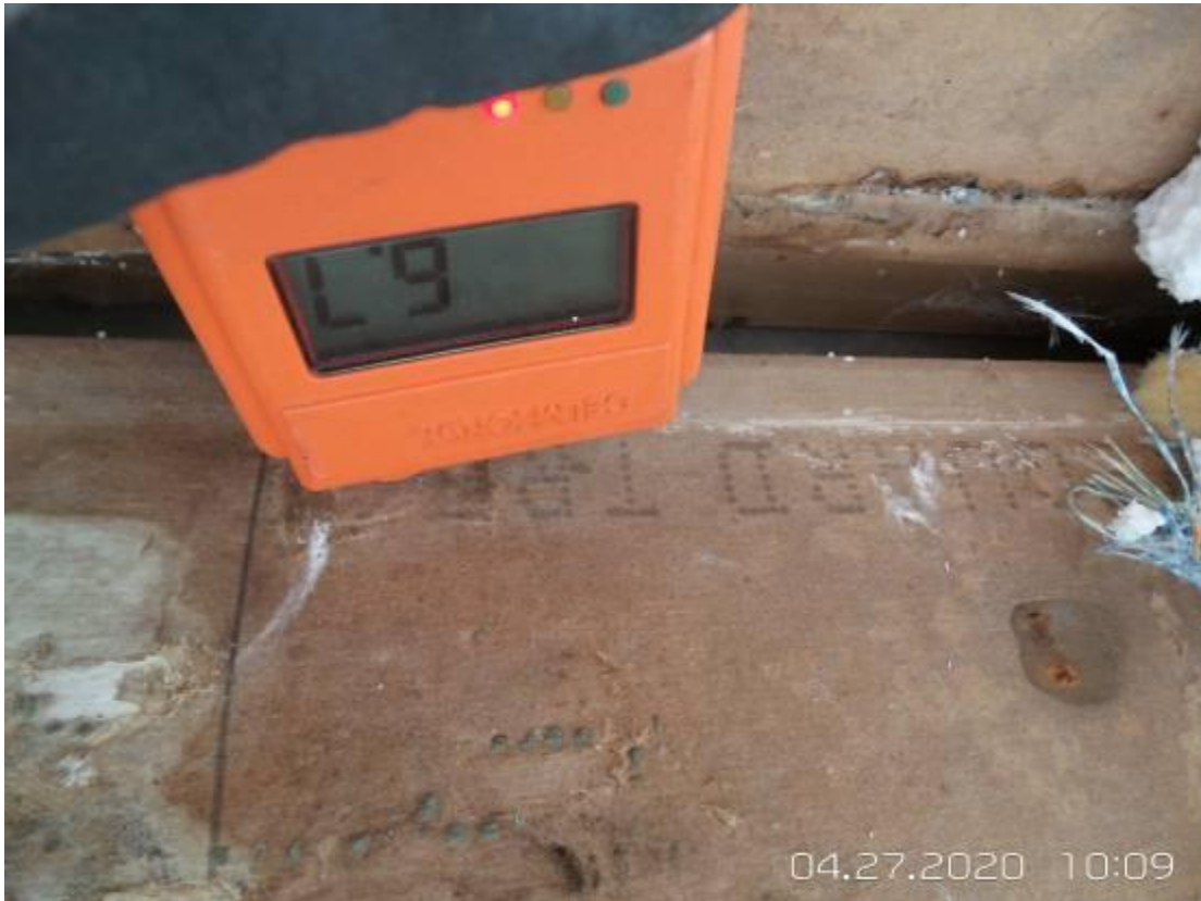
39. Opening 4 – moisture content readings of the gypsum sheathing were normal to wet (0.1% - 6.7%).
