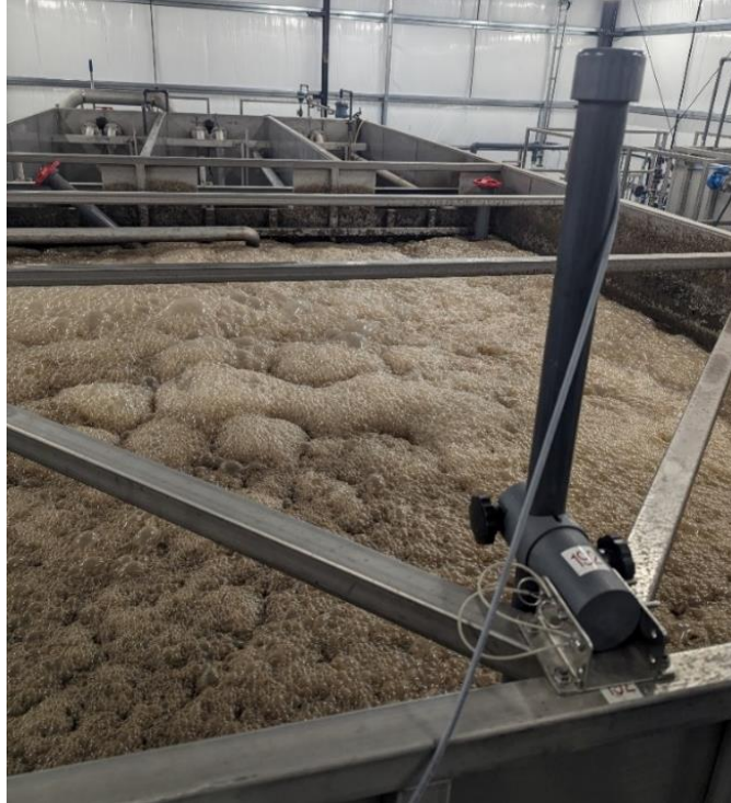
Image 3: MBR Processing Tanks within Treatment Facility
