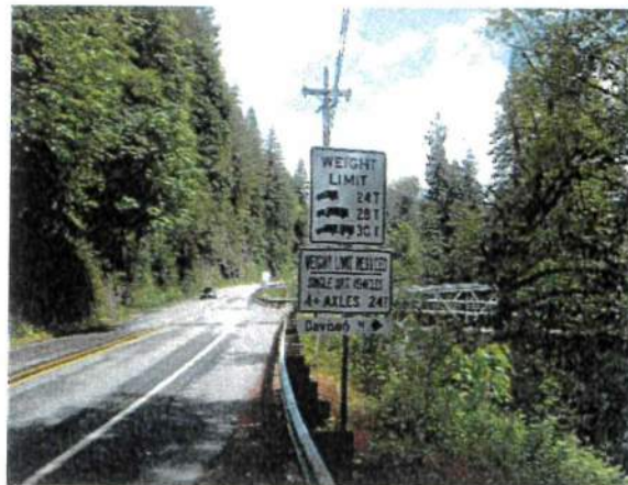
Davison Bridge #1 is posted with weight restrictions
