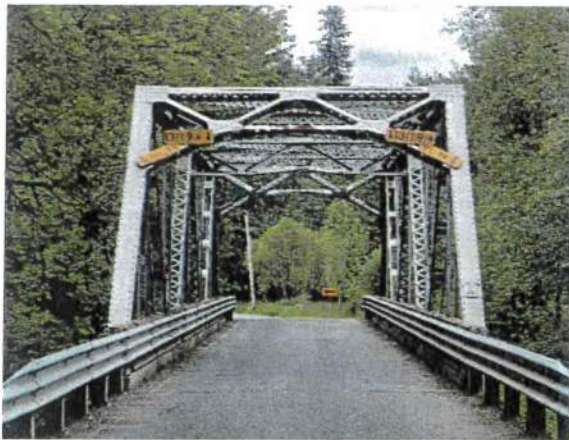
Ferrier Bridge #93 is posted with height restrictions
