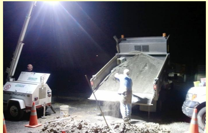
Lewis County Area 3 Technician/WTPO Fred Terry working on the repair at 528 6 th St on the evening of May 19, 2012.
