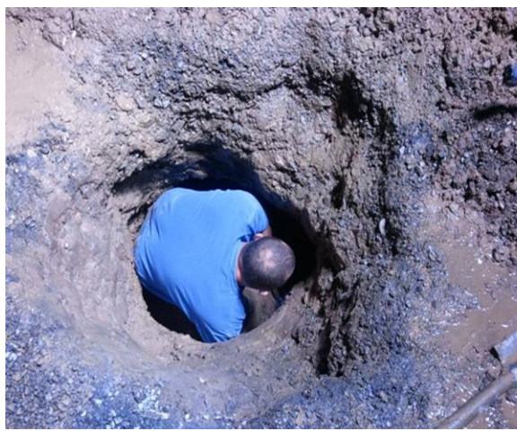
Lewis County Area 3 Technician/WTPO Fred Terry repairing the broken service connection for 528 6 th St on May 19, 2012.
