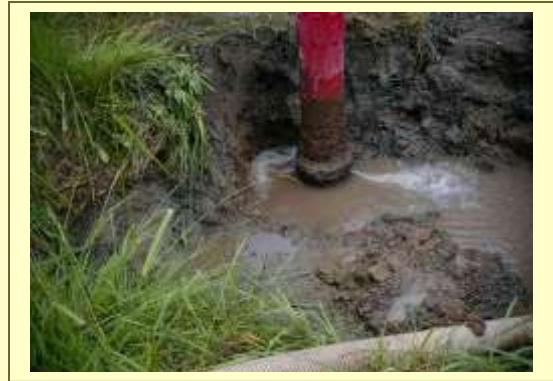
Leaking hydrant at 7 th & A St.
