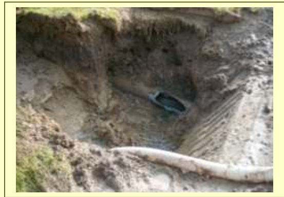
A picture of the burst pipe
